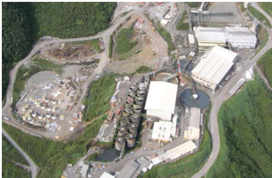
Construction of the pyrite removal section of the mill at the Ok Tedi site.
