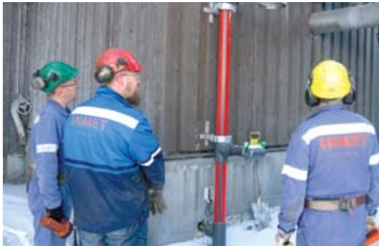
Inspecting and testing a new safety shower near the chemical handling facilities at the Pyhäsalmi concentrator.
